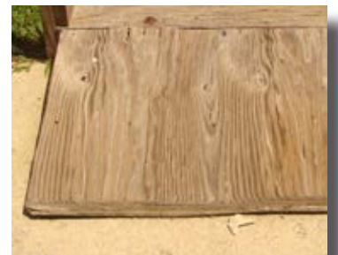
Warped and peeling surface, inch high bump to enter/exit ramp.
